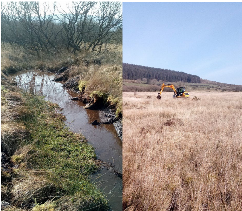
Figures 6 and 7. Blaencleddau. A silt trap pool at the lowest end of a restored stream and view of the machine on site (the stream is entirely lost in dense vegetation and has become piped).
