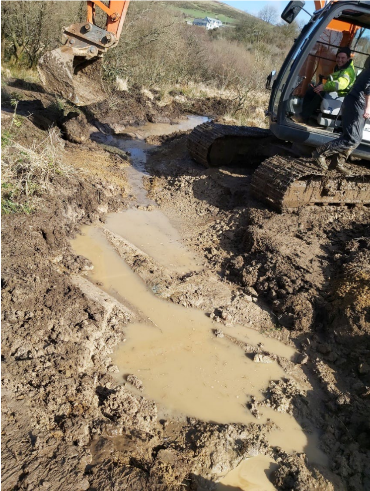
Figure 3. Waun Isaf. Working on the area where the footpath crosses the stream to create habitat and improve access.
