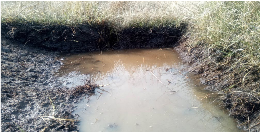
Figure 9. Dolau Isaf. A piped stream with no suitable habitat being restored to a shallow and wide profile.
