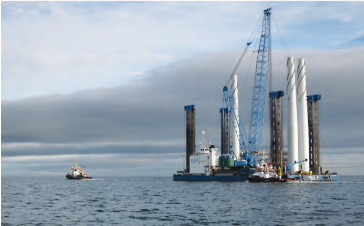
Figure 4 Windfarm jack up rig outward bound under tow from the port of Mostyn through the Mostyn Operational Area.
