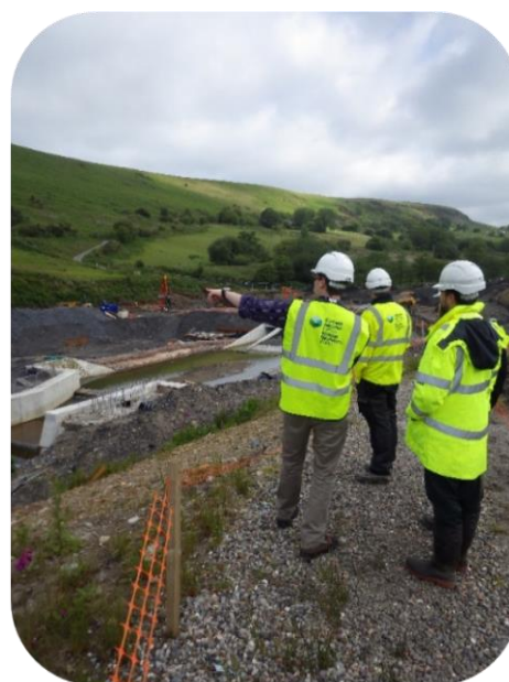
Fig. 7-1: Construction of a new reservoir to store flood water; protecting people from flooding.
