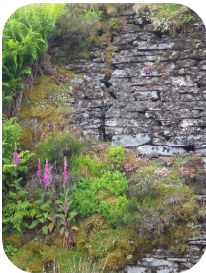
Figure 9-1: Old dams, newly registered will require substantial investment and work by undertakers to bring them up to a safe standard.
