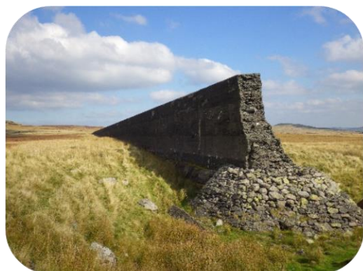
Figure 9-4: A breach in Llyn Eigiau’s dam, above Dolgarrog
