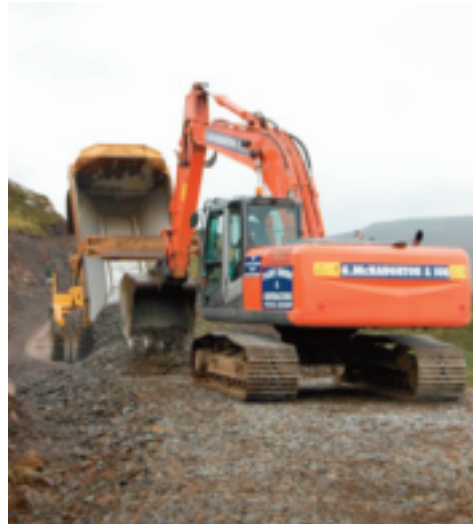
An on-site stone crusher provides material for constructing this forest road on Mull.
