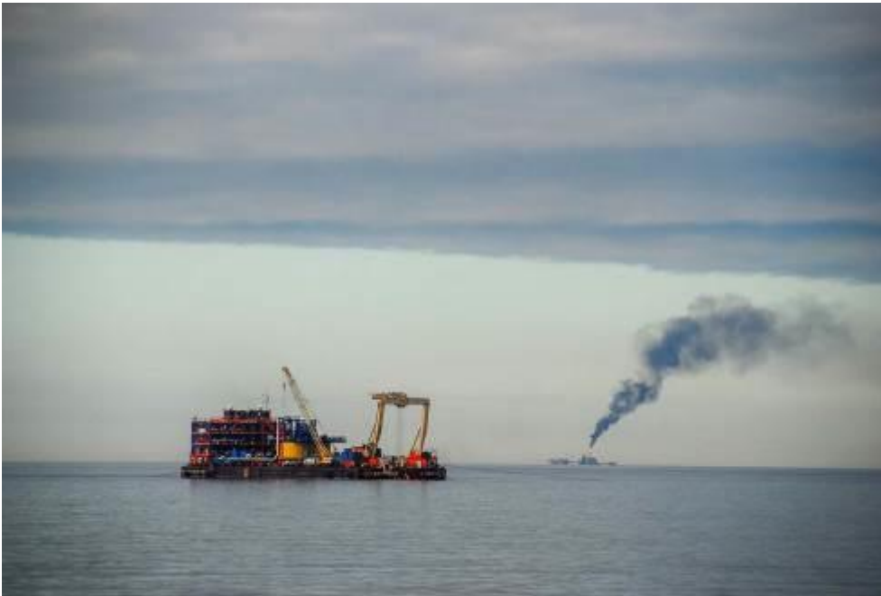
Douglas Oil Platform flare and wind farm construction vessel © John Briggs
