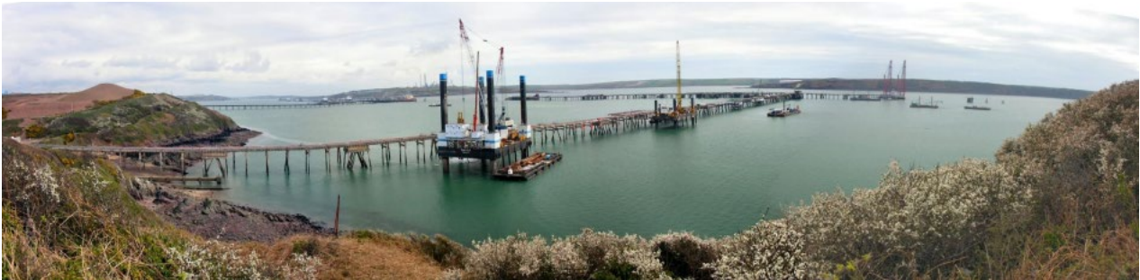
Figure 9: Scale of refurbishment of the South Hook LNG jetty. Photo: Mike Camplin (April, 2006).
